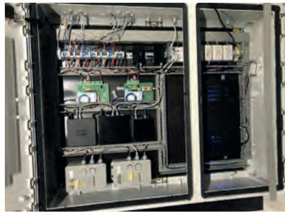
ISLIDE CONTROLLER All products are controlled by iSlide's Control System.
